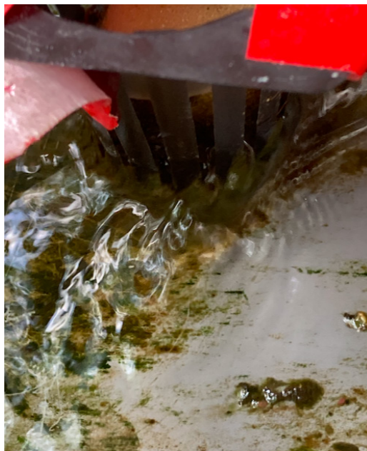
Figure 14. The large biomatter buildup that suffocated Plant 7 in the Pipe System. Note how the biomatter is clogging the basket.
