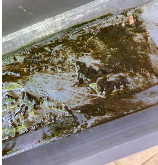
Figure 13. Biomatter in the Pipe System carried by pump. A mix of fish feces, algae and leaves that had fallen in.
